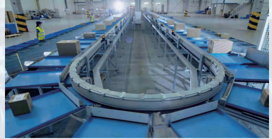
Logistics conveyor line
